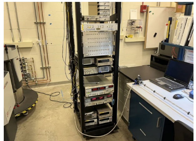
Figure 3: rack positioned to allow lab emergency exit.
