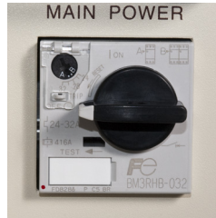
FIGURE 3-15 Compressor main power switch in off position
